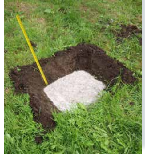
Fill with concrete leaving a depth of e.g. 25/40 cm (see the following pages). Dry for approx. 6-7 days.
